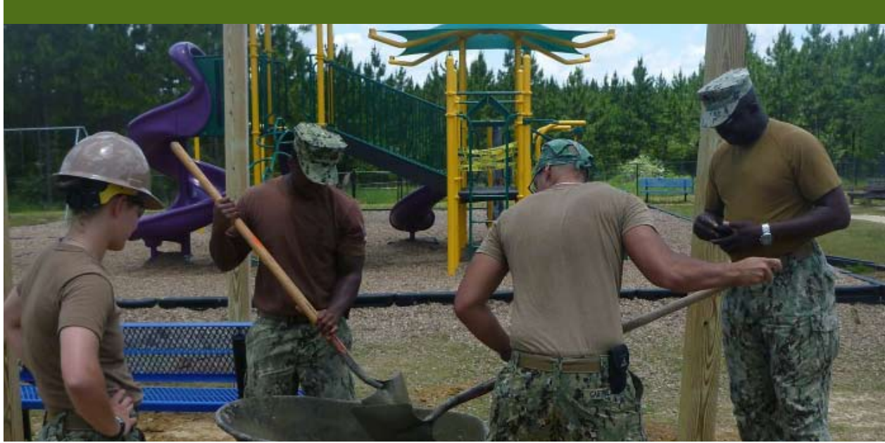
In May, NAVOCEANO employee Michael Bendzlowicz teamed up with a group of Seabees from MCB 133 stationed at the Naval Construction Battalion Center in Gulfport to construct much needed shade over a playground at West Hancock Elementary in Kiln, Miss. Photo courtesy of Naval Oceanographic Office Public Affairs
